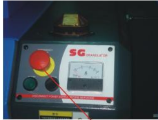
Emergency stop button
